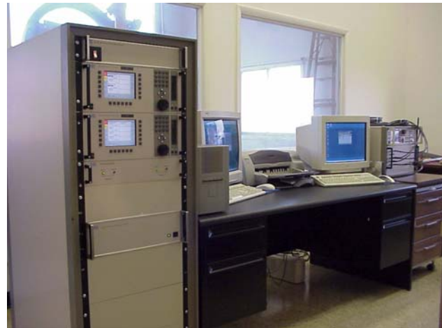
Figure 6. Control Room Equipment
